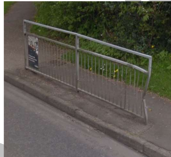
10. A good example of where guardrail could be considered for removal (Gallows Hill Lane, Abbots Langley).
