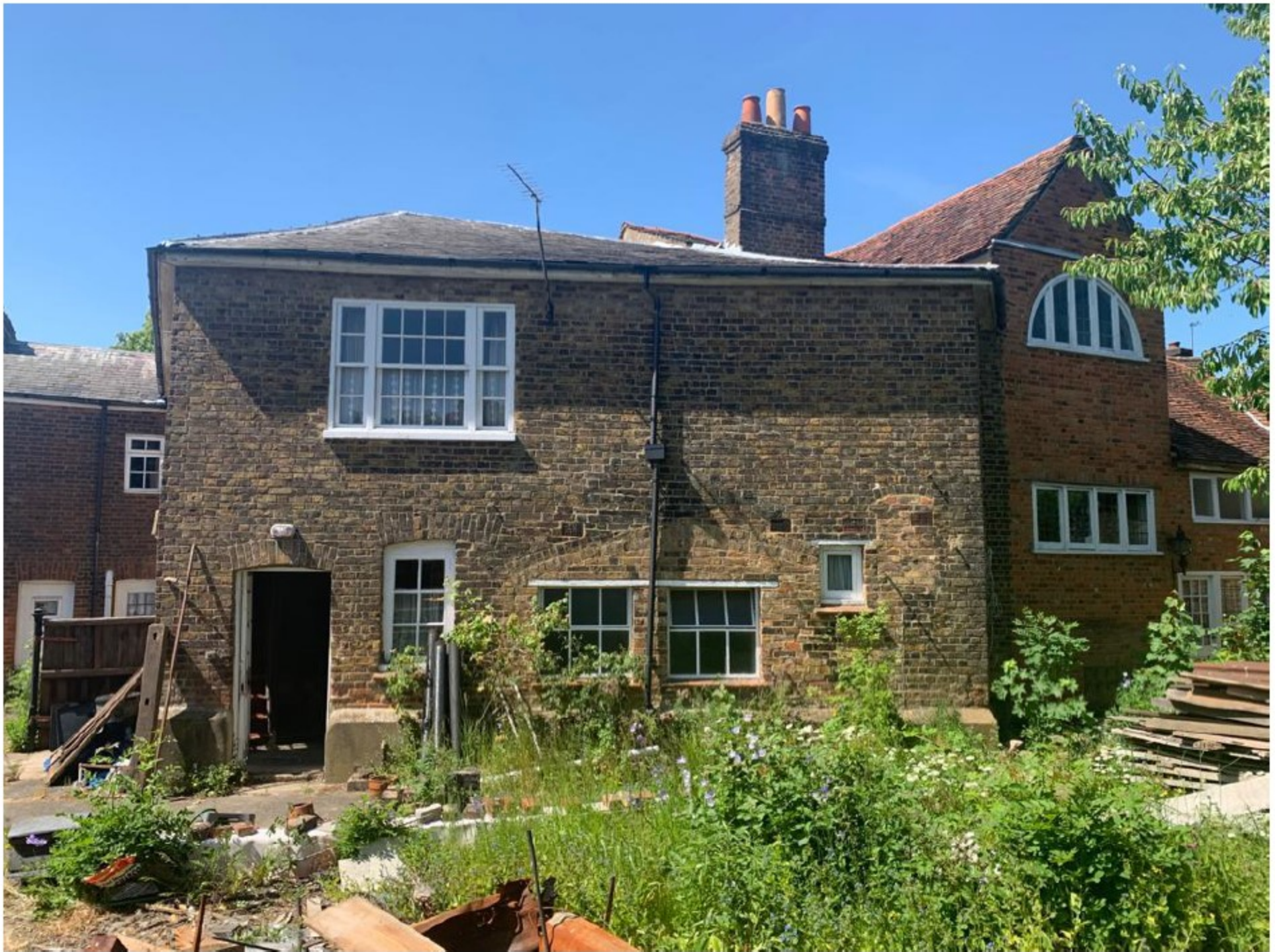
Rear of No 27 with No 31 to the left and No 25 to the right
