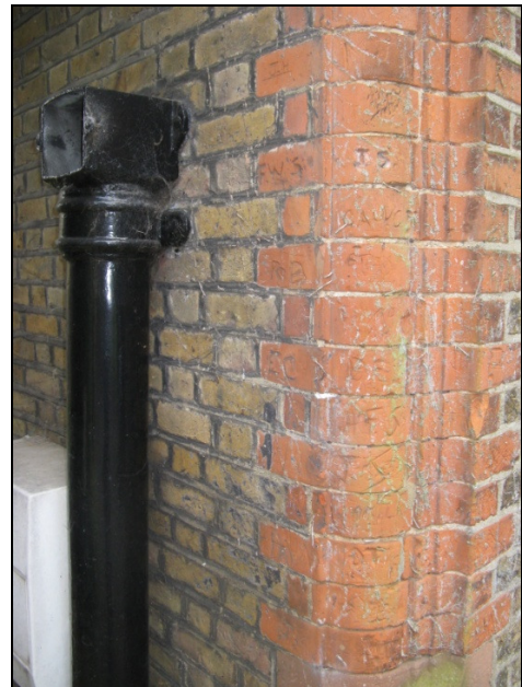
Figure 17 - The historical cast iron drain, and the quoins which have been carved over generations with people's initials.
