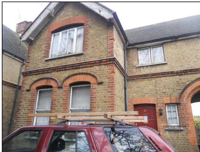
Figure 35 - No. 22, showing the poor condition of the window frames and the inappropriate alterations to the glazing.
