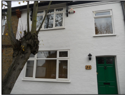
Figure 36 - No. 26, showing the painted exterior and the entirely inappropriate replacement of the window.
