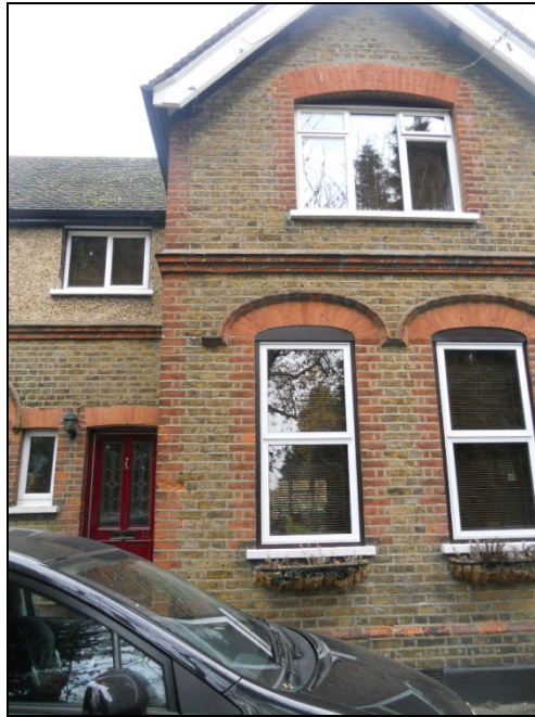
Figure 34 - No. 14 Dickinson Square, showing the inappropriate replacement windows.
