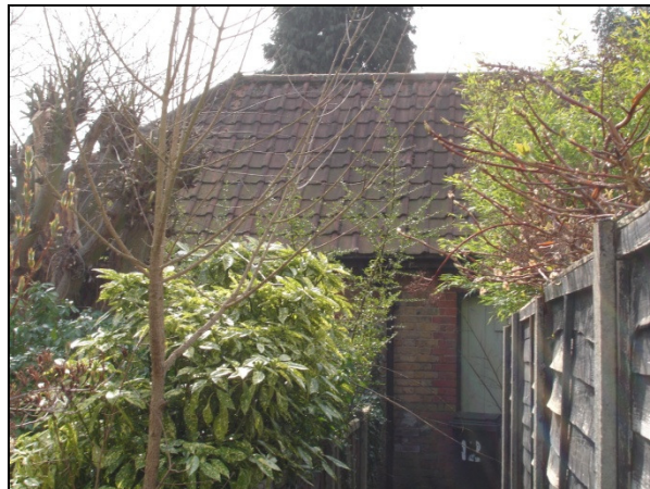
Figure 27 - The small outhouse to the rear of the south side of the square.
