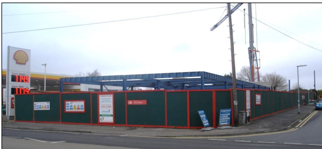
Site under development on Watford Road at the corner of Winton Approach
