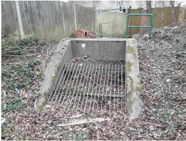
Large drainage inflow
