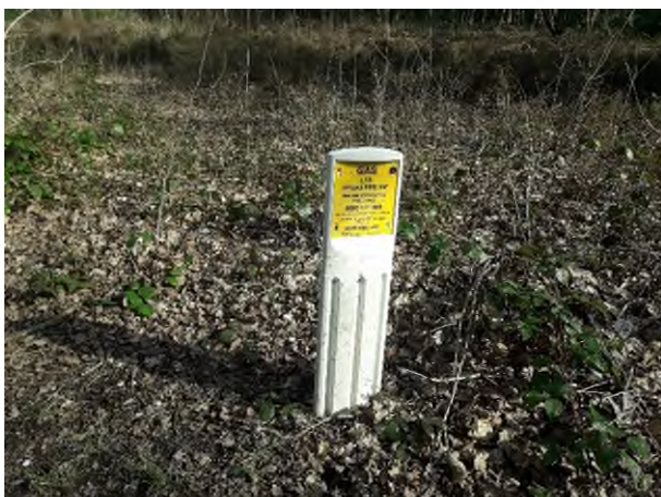
Gas pipeline marker
