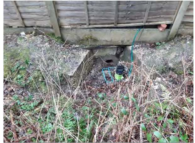
Small drain inflow causing flooding issues
